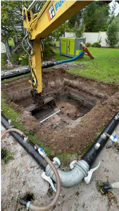
Commencement of the system install at a property requiring the ground water to be lowered (dewatering)
